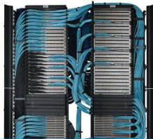
Copper & Fibre Structured Cabling
